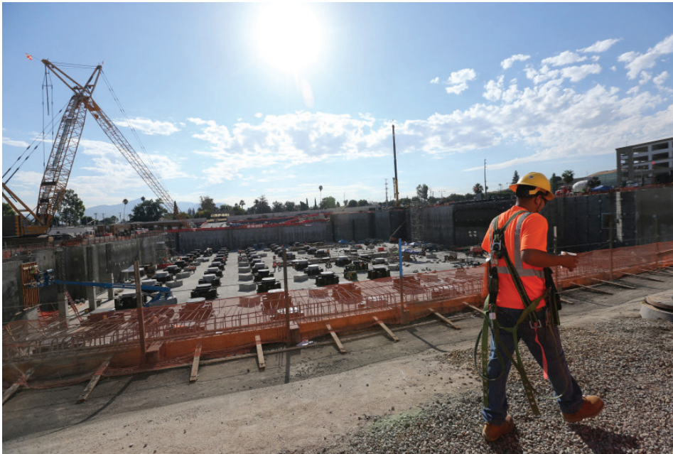
A construction worker walks around the site of the new Loma Linda University Medical Center in Loma Linda on Tuesday, Aug. 29, 2017. The hospital is being built on an earthquake protection system, being the world's first 3D seismically isolated hospital building. (Stan Lim, The Press-Enterprise/SCNG)
